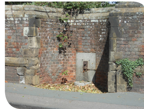
Drinking fountain in the park wall
