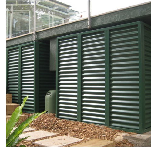
Figure 93: Concealed tanks integrated with the design.
