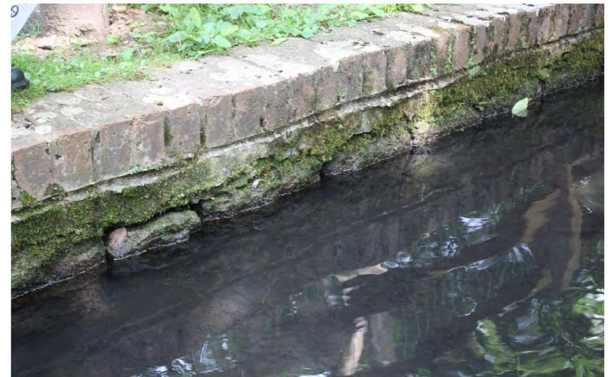
Repairs to stonework required
