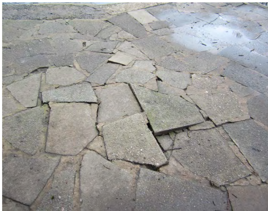
Hazardous crazy paving in need of repair
