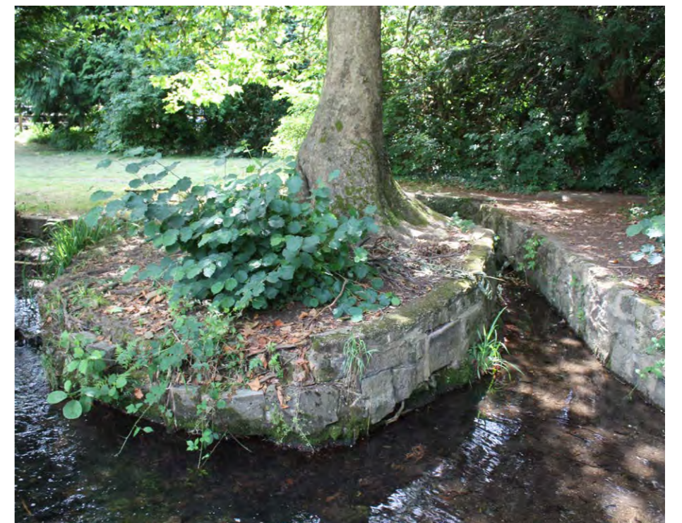
Tree roots pushing out stone walls
