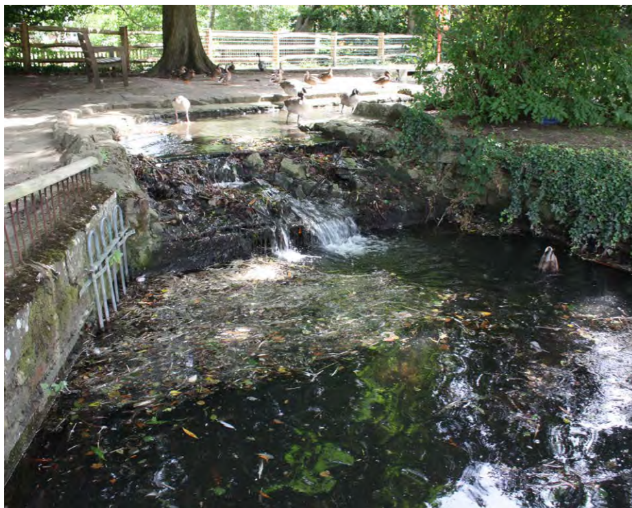
Waterfall wall in need of repair
