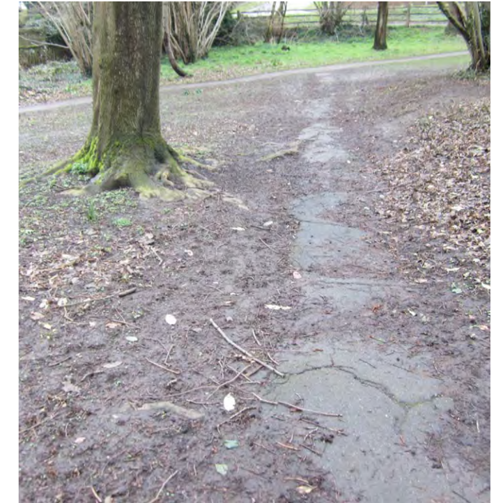
Macadam paths disintegrating
