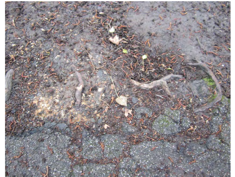
Damage to macadam due to tree roots
